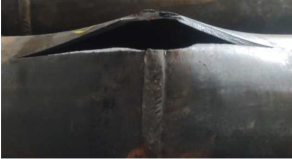
Fig. 6. The damaged area of the pipeline section after the fatigue and burst tests.
